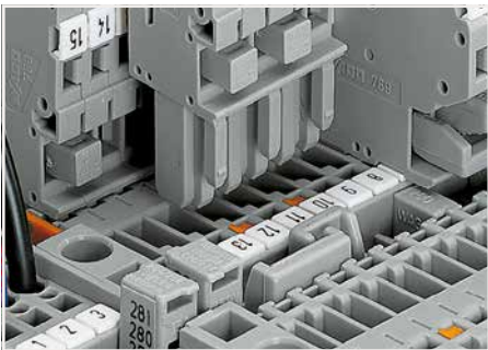
Commoning carrier terminal blocks via staggered jumpers.
