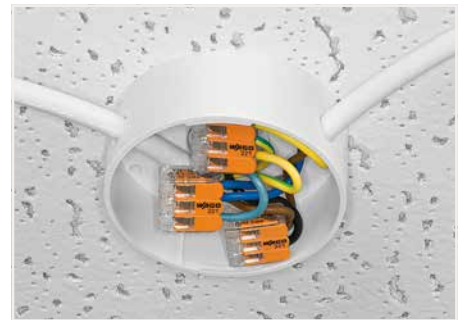
Lighting distribution in a ceiling canopy
